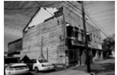
Many buildings seemingly impacted by Hurricane Katrina actually existed in a state of disrepair even before the storm.
